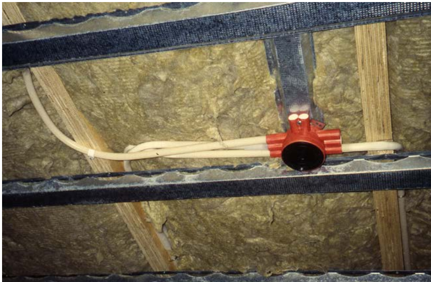
Figure 8.19: a) Typical floor design in timber frame building system. b) Photo of the bottom part of the floor with electric installations.
