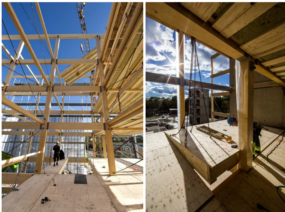
Figure 8.9: a) The post and beam system “Trä8”, Askims torg (Moelven Töreboda). Photo: Sören Håkanlind.
