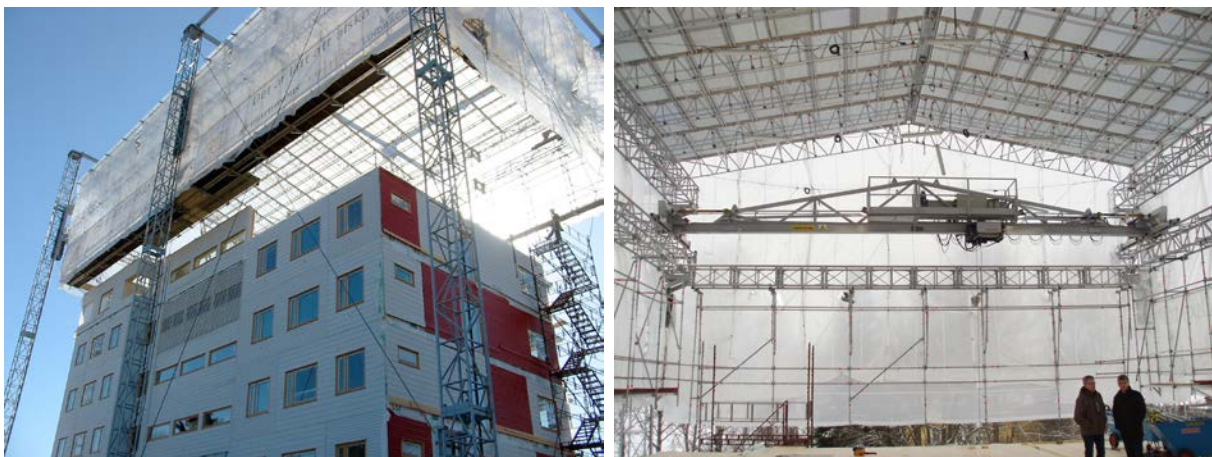
Figure 8.14: a) Movable tent over the whole building. Älvsbacka Strand, Skellefteå, Martinsons Byggsystem, Lindbäcks Bygg AB and White Arkitekter AB (Photo: Anders Björnfot). b) Movable tent from the inside with integrated travelling crane (Photo: Anders Gustafsson).
